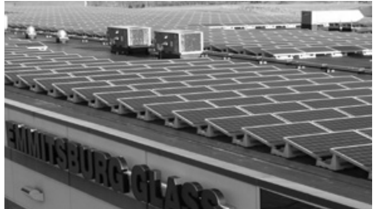
Emmitsburg Glass' solar panels will produce 276,004 kilowatt hours/year, allowing Emmitsburg Glass to go 100% solar.
